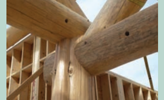
Joinery: This demonstrates the fine joinery of round log to round log by master log builder John Nininger of Newbury, VT and his crew.
