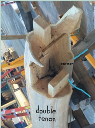
Double tenons: These tenons secured two trusses going in two directions on two levels. Extremely difficult workmanship.
