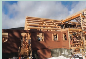
Roof purlins - Roof purlins in place on top of log trusses. Most visible logs came from Put Blodgett's Bradford Tree Farm.
