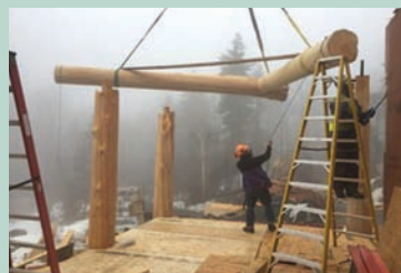
Hoisting logs - Notice tenons on top of uprights to fit into mortises (holes cut to receive tenons)
