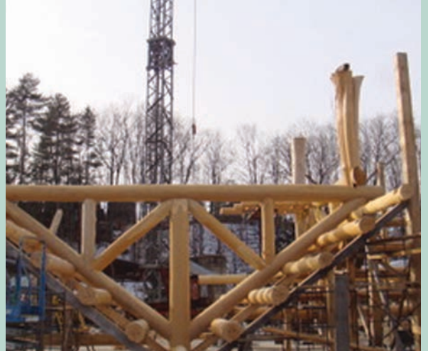
Upside down trusses: The purlins (longitudinal rafters) are shallowly sawed on one side to achieve a flat surface and then that side placed against an upside-down v-frame. This results in a flat roof with the vertical uprights holding up the trusses cut to length to match the diameter of the various trusses.
